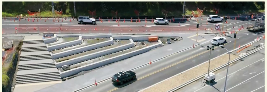
The new retaining walls on the corner of Church Road and Lagoon Drive.
