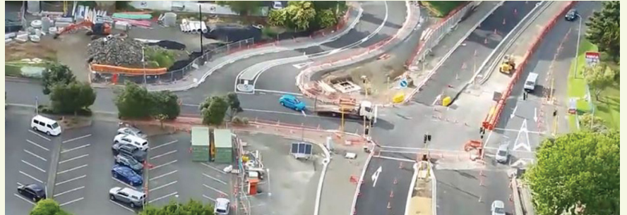
Eastbound traffic is using the new busway, which allows work to continue along the centre of Lagoon Drive.
