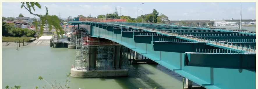
The busway bridge has arrived on the Western Abutment. The prefabricated concrete on the busway is placed over steel girders to create the road.
